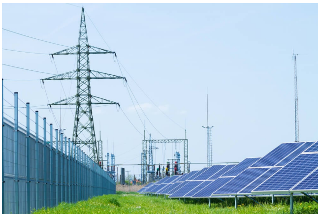
A fully remote microgrid has disadvantages: There are no benefits from grid supply. Thus, the project owner needs to invest in assets to support the entire facility
